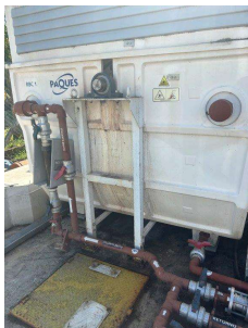
Foto 3 - Módulo RBC - rotating biological contactors
